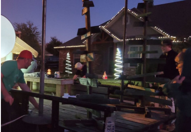
Building the float in front of our President Lion Mandy Moss' house
